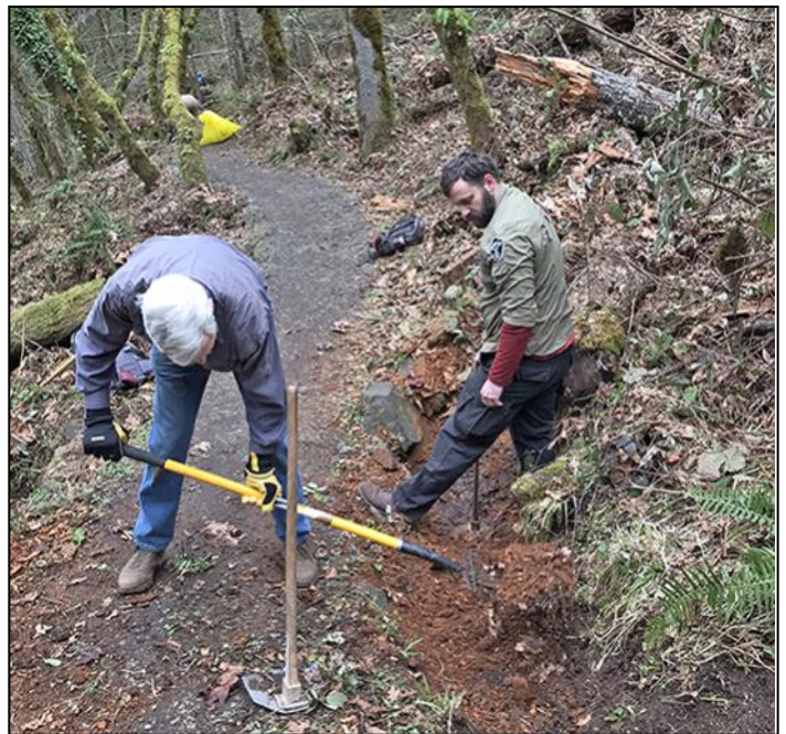
Larry clears the drainage area while Matt works on the culvert opening.
