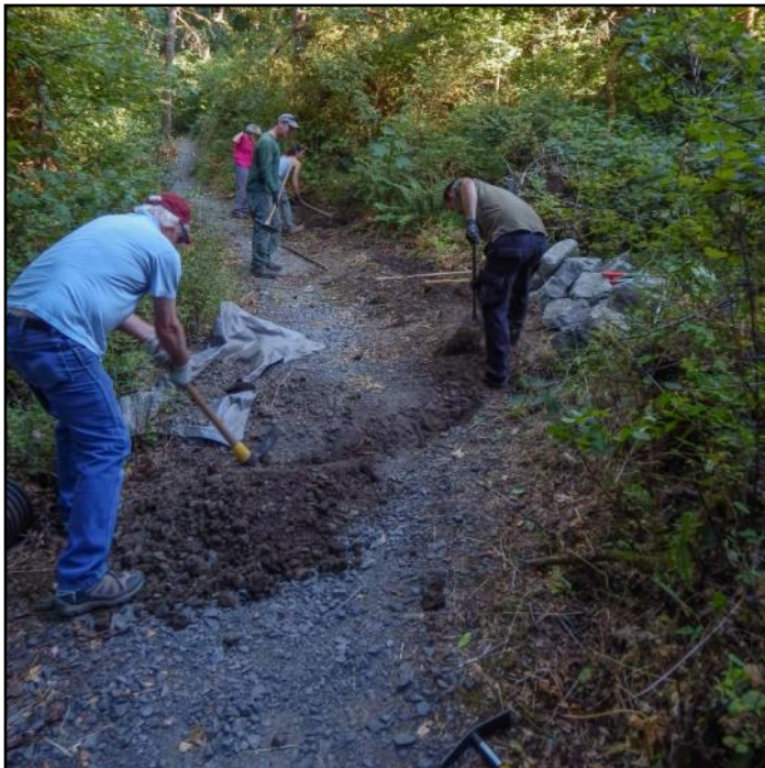
Dan and Matt work on the culvert ditch while Dev, Brianna and Janet tackle the drainage ditch.
