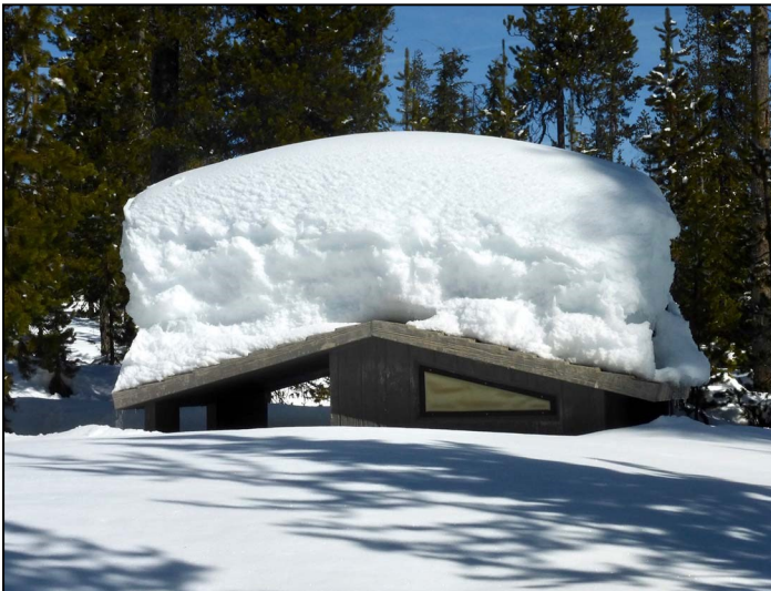
Does this look like a restroom? At least 10 feet on the roof.
