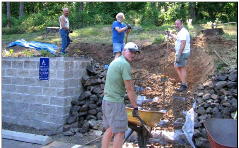
Speaking of hot summer activities, five stalwart grounds crew members recently completed the hand excavation of the steps to ease access to the rear storage areas at the Lodge on a 90+ degree afternoon. From the left, Doug Nelson, Gary Kirk, Stewart Hoeg and John Jacobsen. Jim Pierce, another stalwart hot weather digger, snapped the photo.
