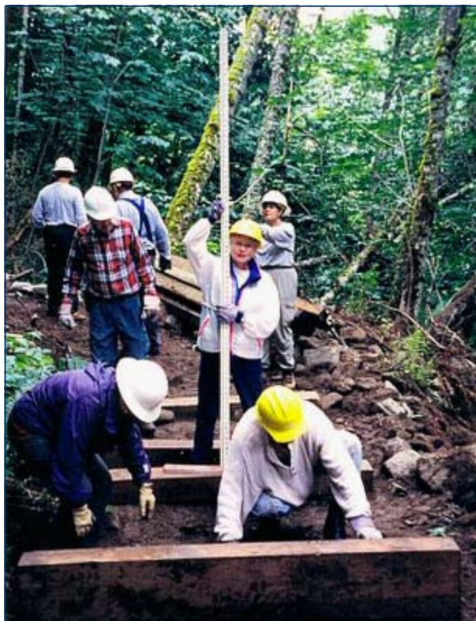
Ann Bonine, center, holding survey rod. Beginning stages of building a low bridge. Goat Trail, Steven's Pass, WA, July 2003, with the American Hiking Society.
