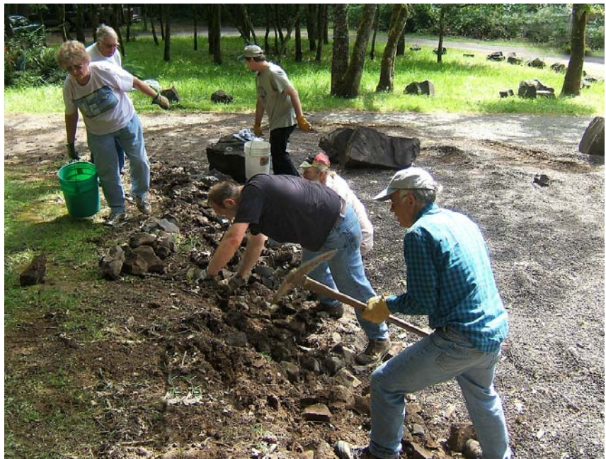
Rock wall coming down. Clockwise from left: Joella, John M, Rick, Wayne, John J, & Richard.
